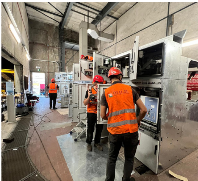
Quadri di primaria installati in Acciaierie Cogne Primary electrical panels installed at Acciaierie Cogne
