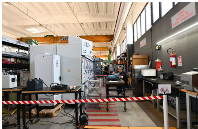
Collaudo quadro elettrico in media tensione Medium voltage switchboard testing
