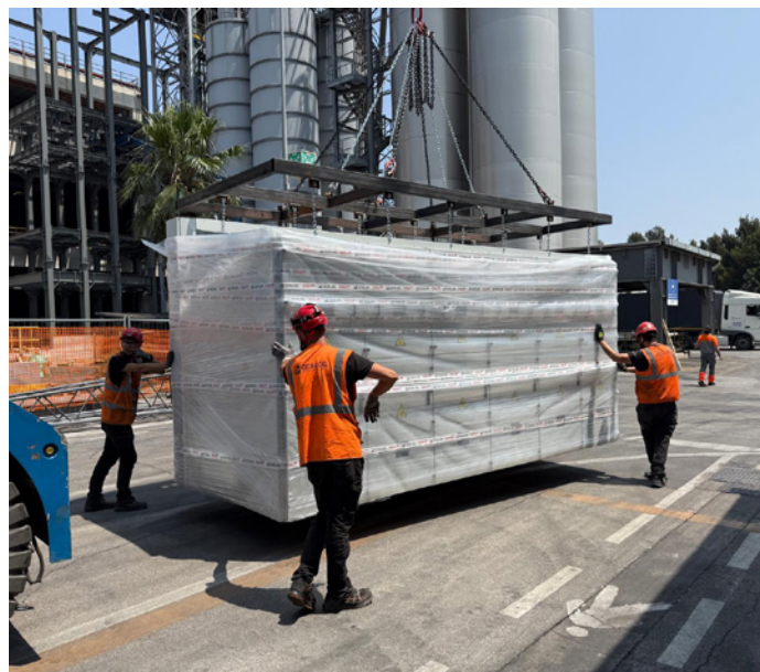
Quadri di primaria installati in Bridgestone Primary electrical panels installed at Bridgestone
