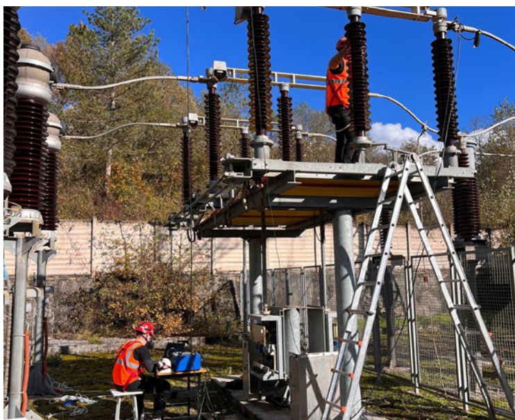
Manutenzione e test apparecchiature in S.S.E. Maintenance and testing of equipment in S.S.E.
