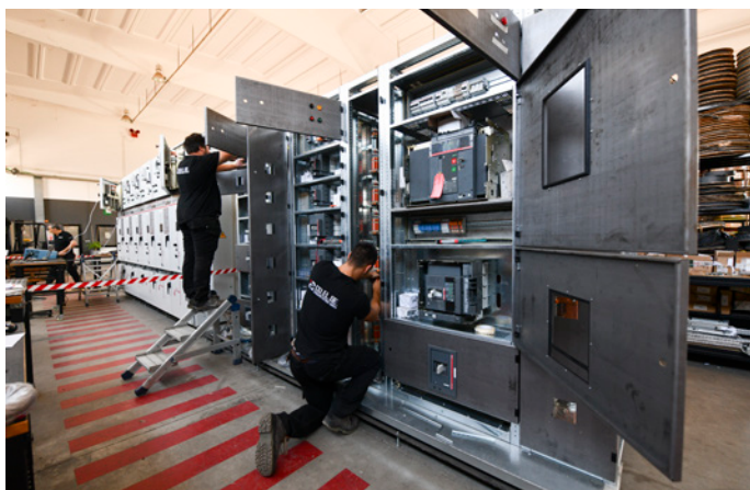
Assemblaggio quadro Power Center Power Centre quad assembly
